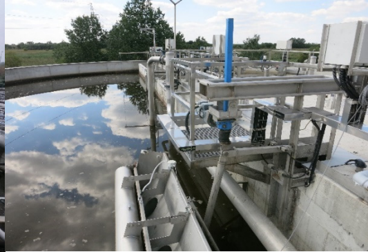
Circular Contiseq™ facility
