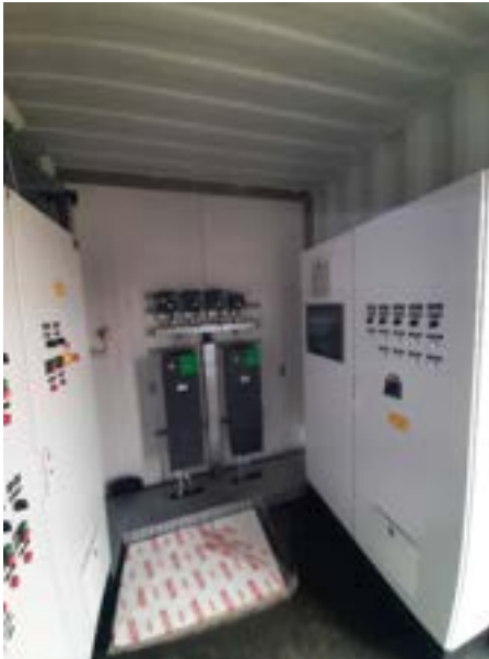
Containerized Electrical Control Room
