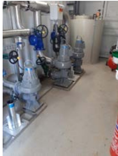
Containerized Equipment Room)
